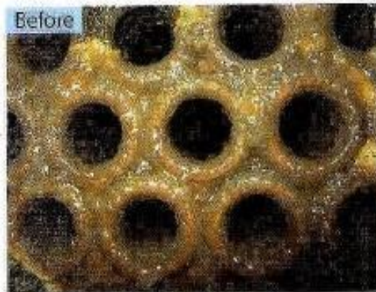
Slime and fouling at heat exchanger
