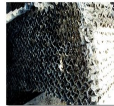
Cooling Tower Infill Fouling
