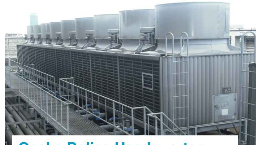
Osaka Police Headquarter Hospital Cooling Towers
