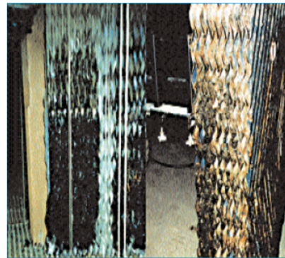
Biological fouling is the root of most cooling-loop water treatment problems, according to many experts.
