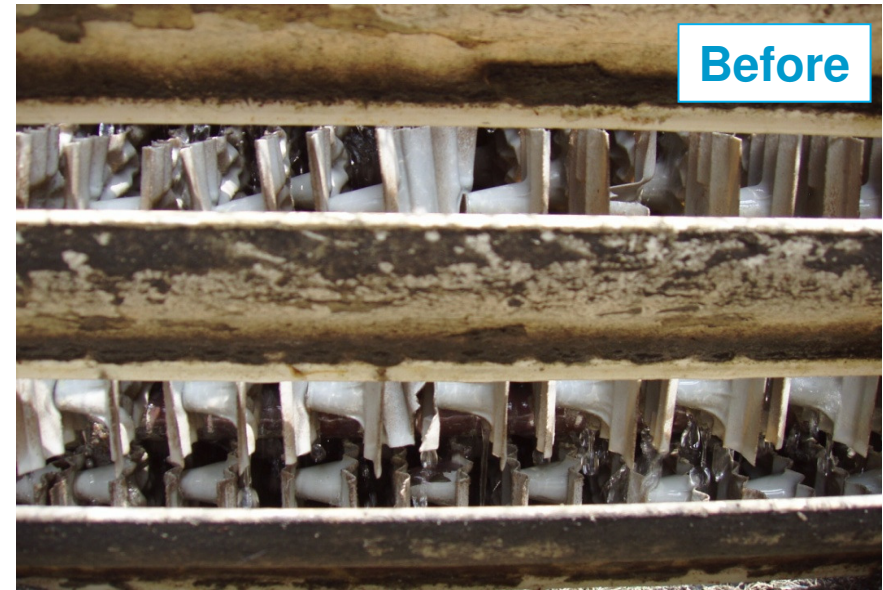
Cooling Tower infill slime and fouling
