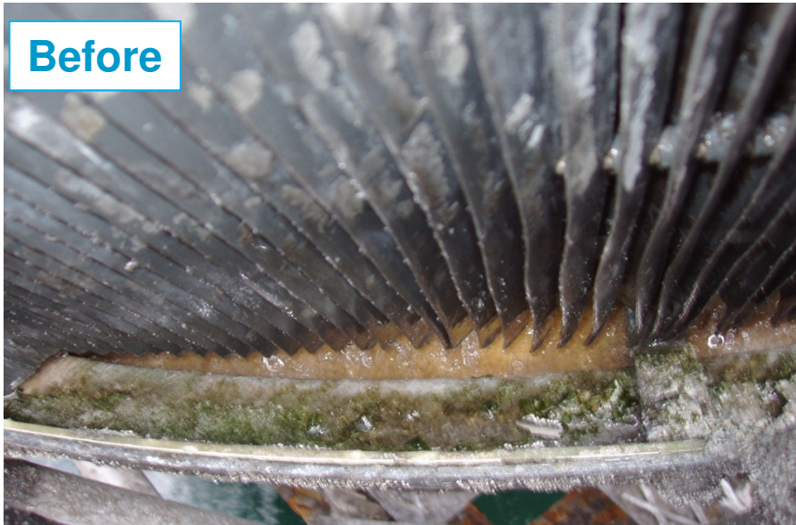
Slime at bottom of cooling tower
